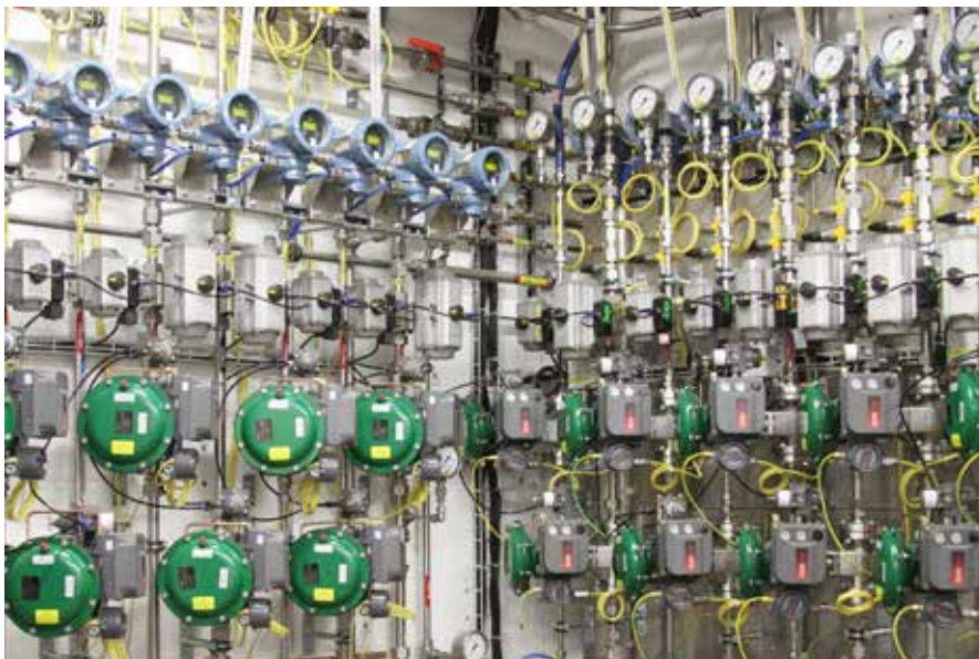
Modern gas supply system in a laboratory
