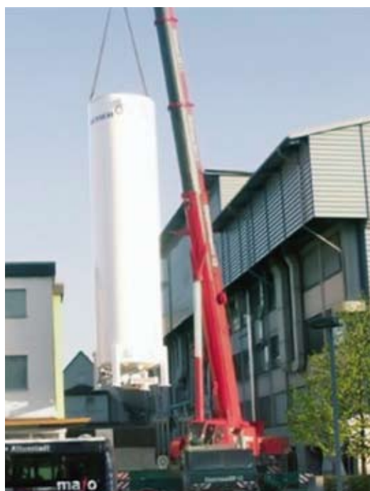
On-site installation of the nitrogen tank at Zeiss
