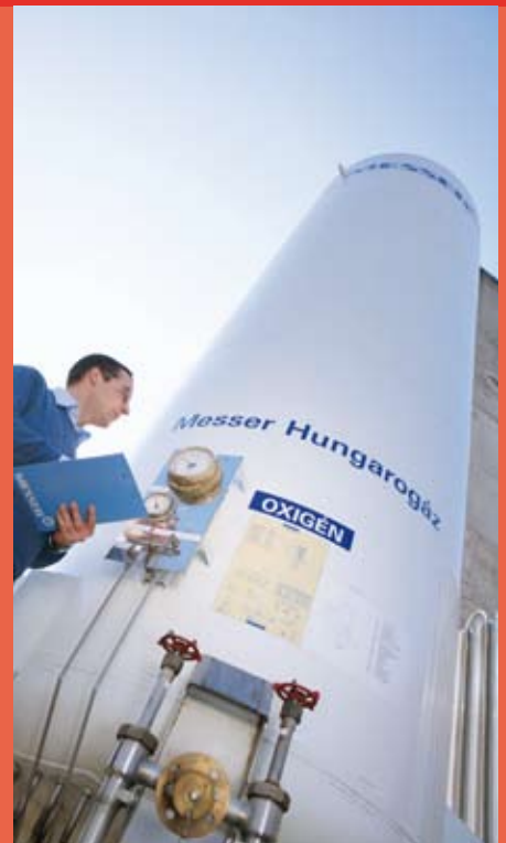
The liquid oxygen is stored in tanks at the customer site.
